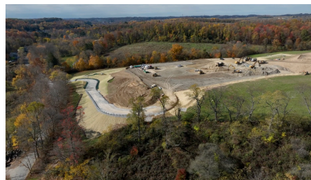
Pictured: Other local well pad being built in Westmoreland County, adjacent to residential property.
